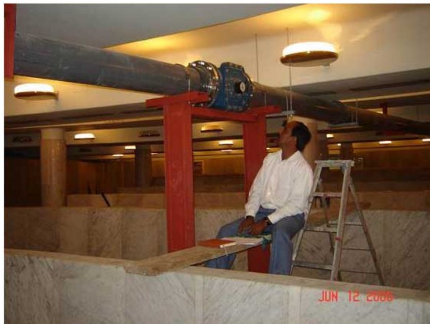
A view of part of water disposal pipe with analogue flowmeter
