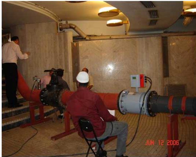
A view of part of water disposal pipe with digital flowmeter
