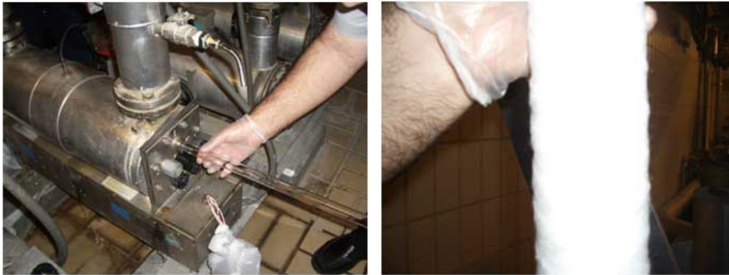
Inspection of quartz sleeve of UV unit Inspection of Clean cartridge Filter
